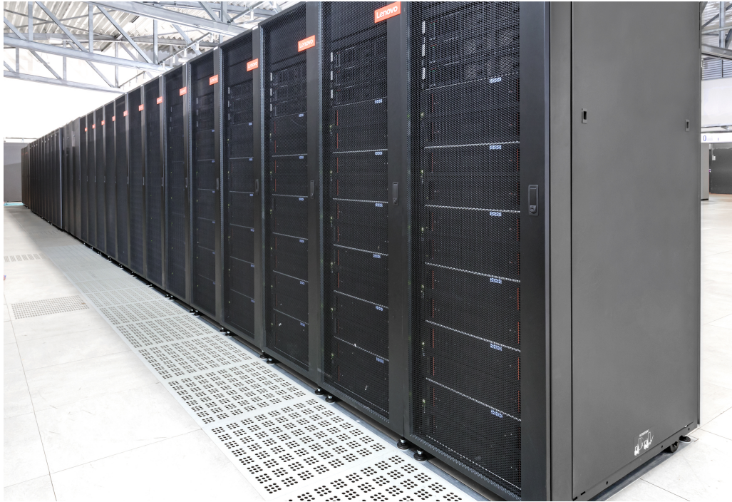
Figure 1: Disk-arrays in the storage cluster JUST in the facility of Jülich Supercomputing Centre. Copyright: Forschungszentrum Jülich GmbH.
